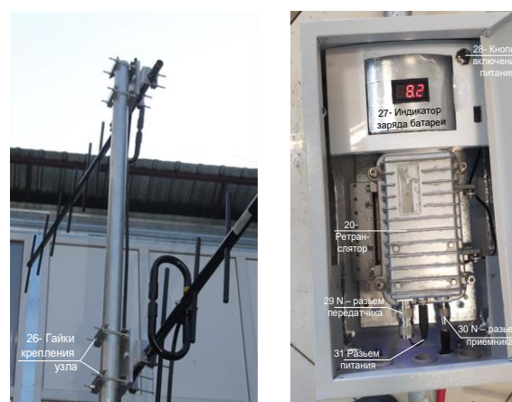
a) receiving antenna at the top and transmitting antenna at the bottom of the mast
